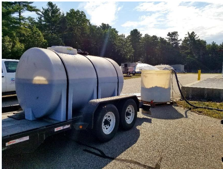
Figure 2: Sludge supply setup during WAS trial
